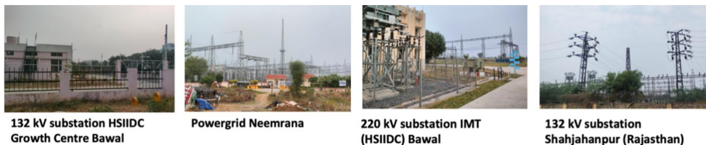
Figure 11: Snapshot of the various substations visited
